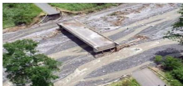
Remains of Bridge near Popenetta.
