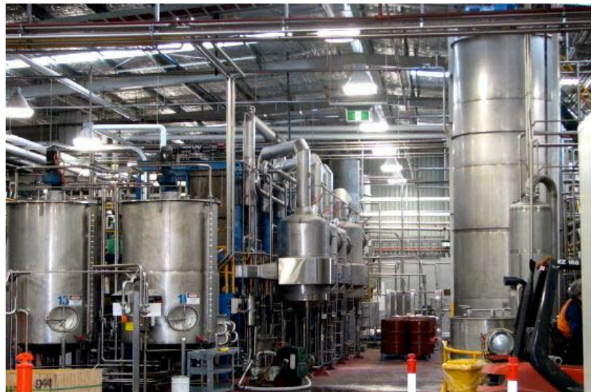
The view inside the newly rebuilt Mildura Fruit Juice Company, where the machinery is new and gleaming and laid out in an efficient manner.
